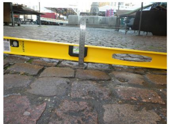
Photo 20: Undulation of 20mm on walkway in zone 3.
