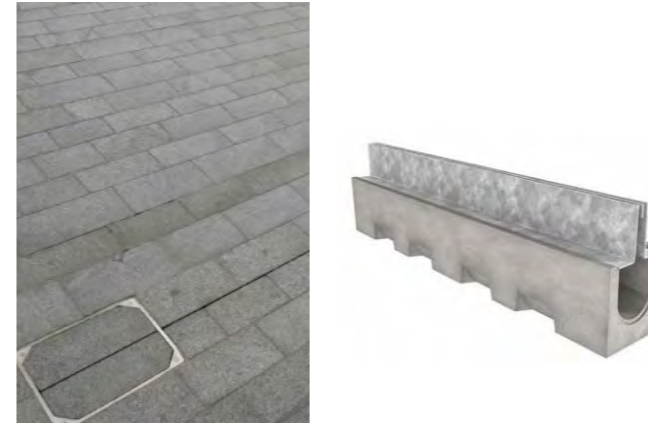
Slot channel maintenance access
