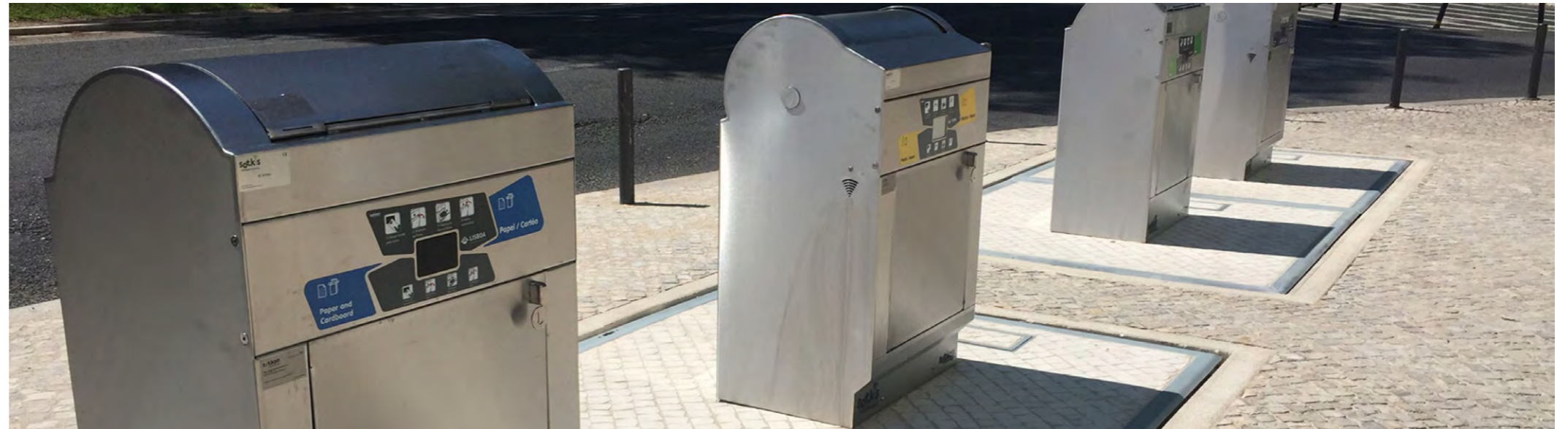
An example of a below ground waste management system with PAYT chip readers and rear access hatches for bulkier waste
