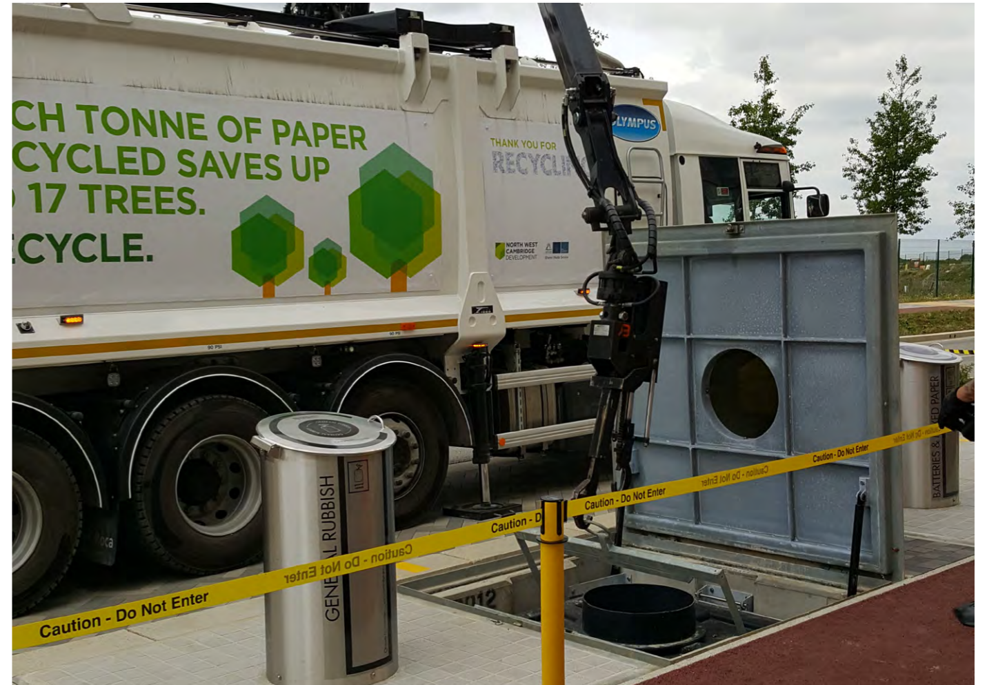
Example of underground waste system at Eddington, West Cambridge
