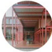
Exposed Steelwork: Expressed steel structure with matte red colour. Opportunity to reuse steel from donor building.
