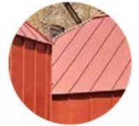
Standing Seam Roofing: Standing seam roof in pastel red colour. Seams to align with primary steel frame direction.
